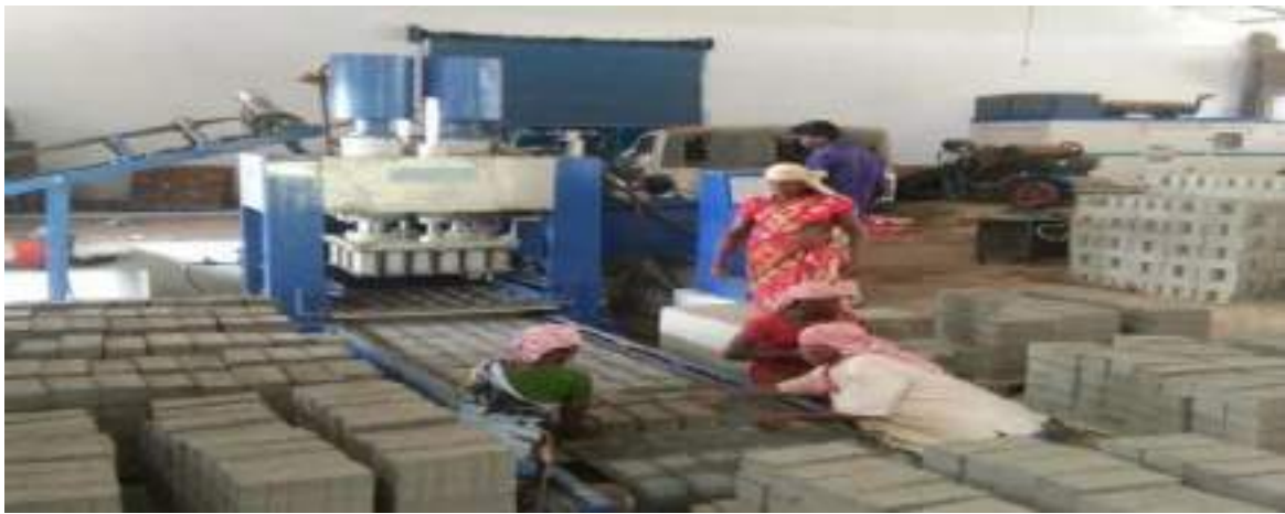
Fly ash brick manufacturing plant at M/s B S Sponge Ltd Raigarh
